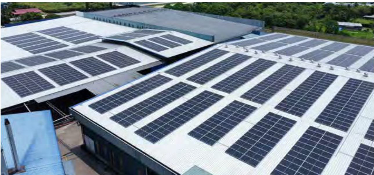
Sky view of Sungai Bakap Factory with solar panel installation
